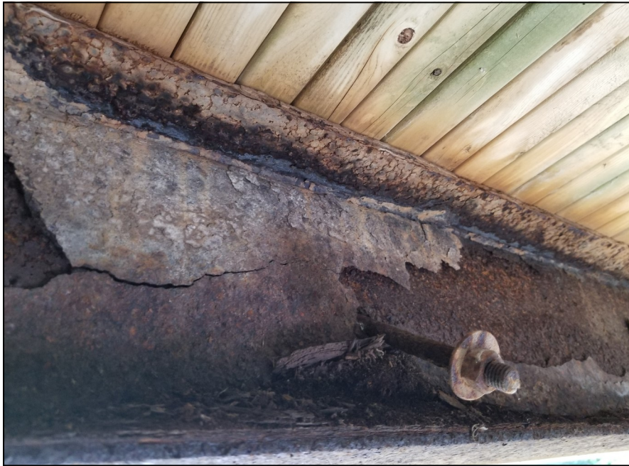
Photo 15 - Approximately 30% section loss throughout stringer supports (September 22, 2020).
