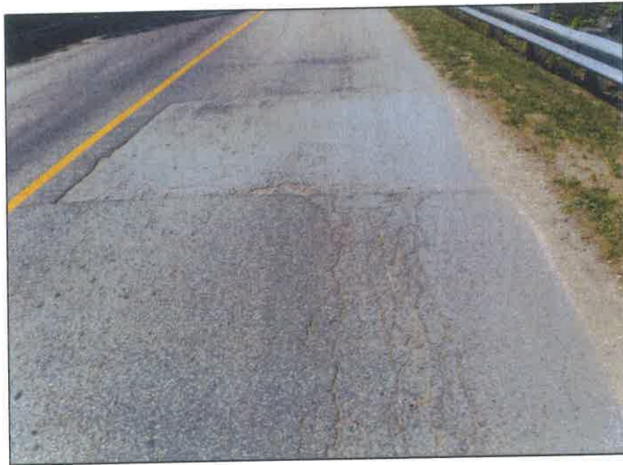
Photo 3 - View of cracks and patch in asphalt.
