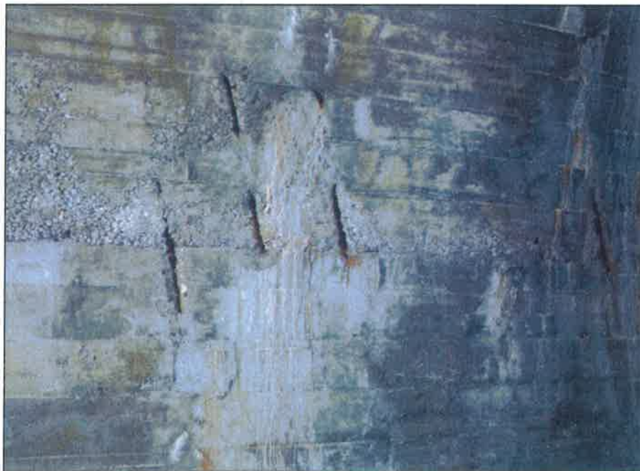
Photo 6 - View of typical efflorescence and exposed rebar in barrel wall.
