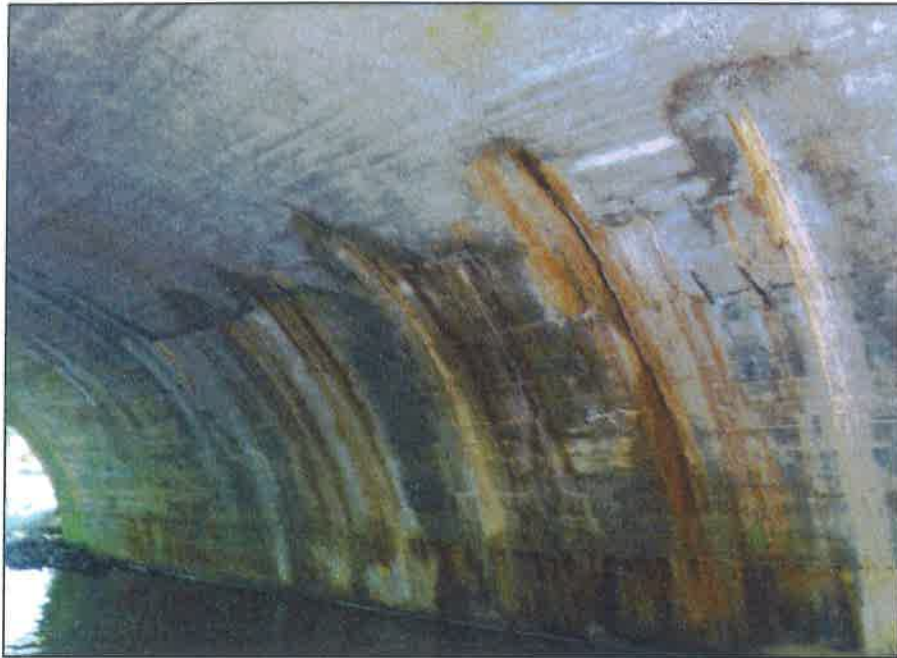
Photo 5 - View of typical staining and leaking in barrel wall.
