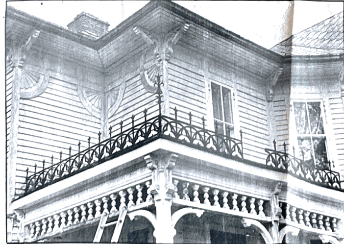
ARCHITECTURAL SIGNIFICANCE —The iron cresting along the top of the veranda is being replaced, as well as the spindles and posts along the veranda.
