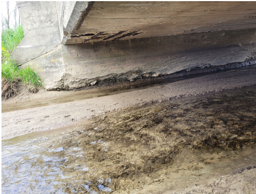
View of erosion under abutment wall, typical.
