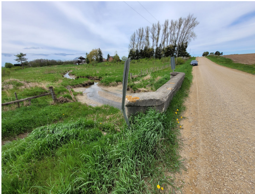
View of damaged southwest hazard sign.
